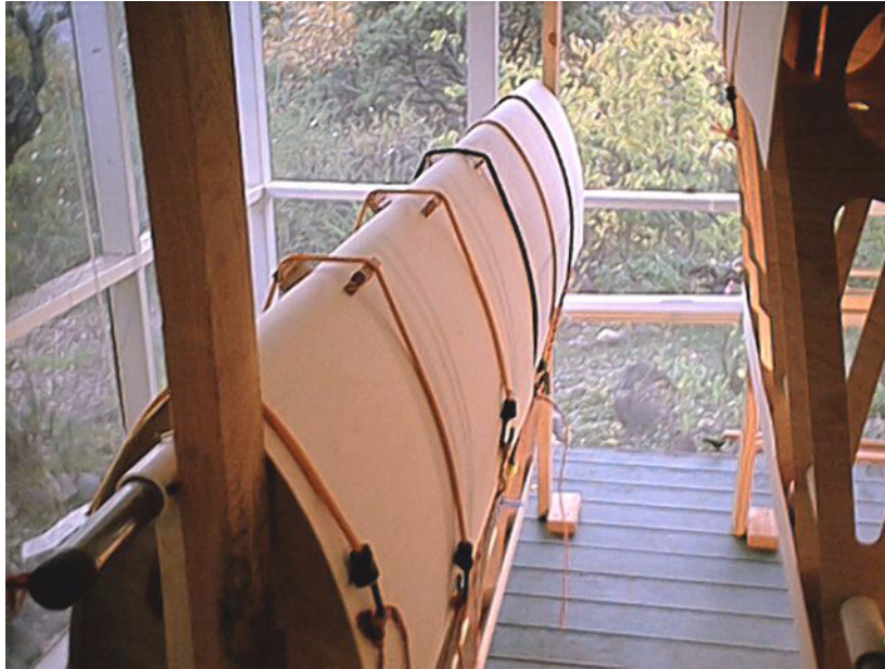
Figure 5-46 Plywood leading edge skin glued to wing ribs. The wing skins suffered severe cracking problems when bent around the leading edge. In order to accommodate the sharp radius of curvature, the wing skins were thinned and soaked in water before gluing them on to the ribs to form the forward “D” tube. This area remained weak and prone to damage in the finished wing structure.
